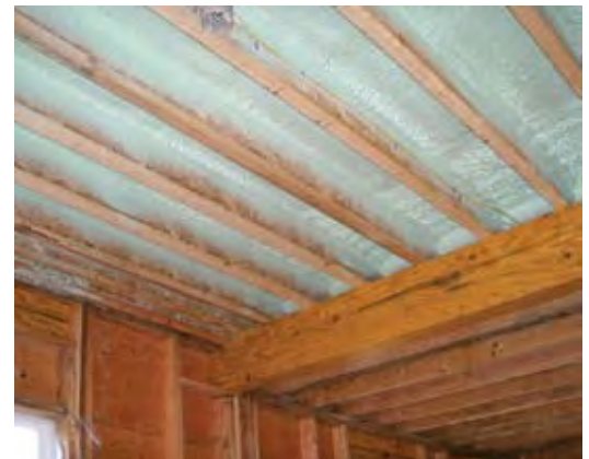
R-6 closed cell spray foam flash seal
