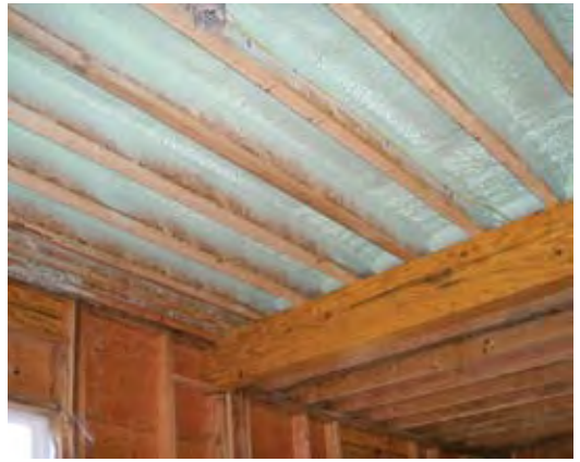
R-6 closed cell spray foam flash seal
